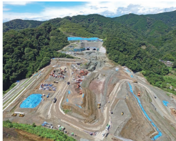
Bird's eye view of Shiozawa section of Kawanishi Project (large-scale banking and tunneling work)
