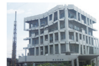
Damage to Uto City Hall
