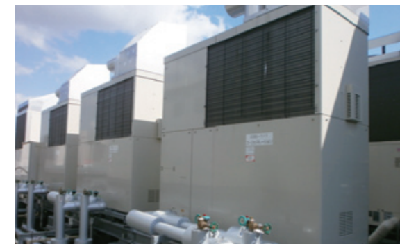
Aizen Hospital Energy Equipment Service (Sapporo) Provision of an energy service that includes installation and maintenance and has no start-up expenses
