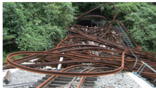
Rails knocked away by the heavy rain and the landslide and blocking the tunnel (immediately after the disaster)
