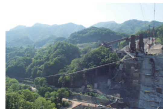
The conveyor belt at Yanba Dam
