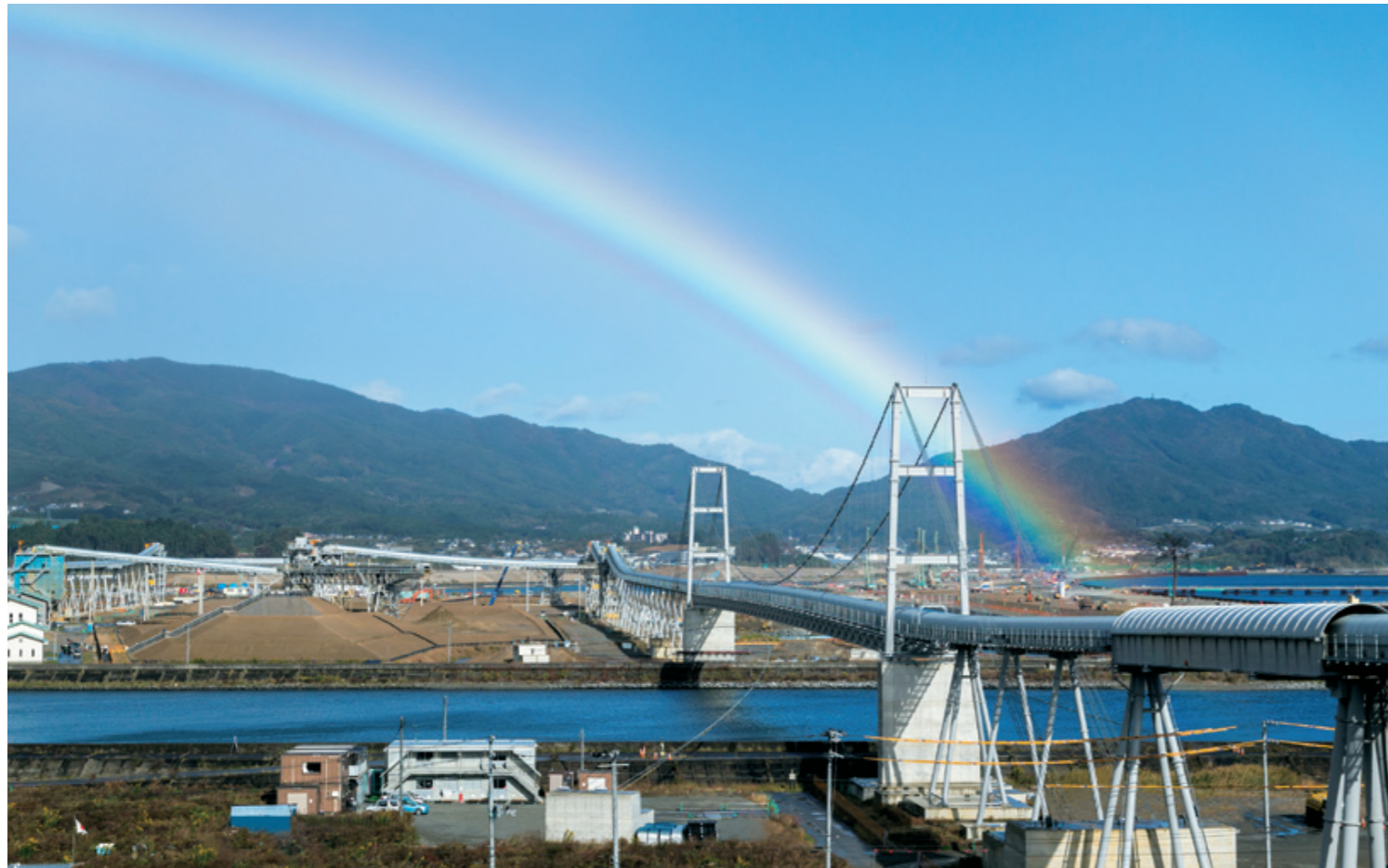
The "Bridge to Hope" at construction sites in the Takata and Imaizumi districts of Rikuzentakata (Iwate prefecture, see page 48)
