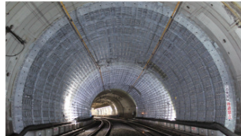
Permanent countermeasure against deformation of railway shield tunnels caused by increased loads: Takashima Tunnel reinforcement construction
