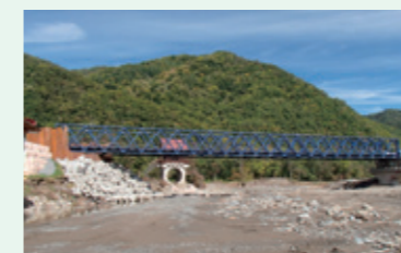
The temporary span at Chiroro Bridge (removed during progress on restoration construction)
