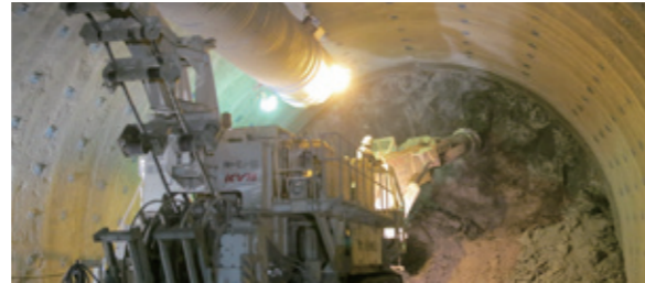
Rising to the challenge of full face mechanical excavation and the immediate ring closure method in weak rock: Hachinoshiri Tunnel, Chubu-Odan Expressway
