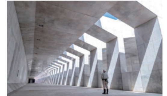
Construction on concrete caisson no. 6 in the Ichikawa-Tajiri zone of the Gaikan Expressway (Ichikawa, Chiba Prefecture)
